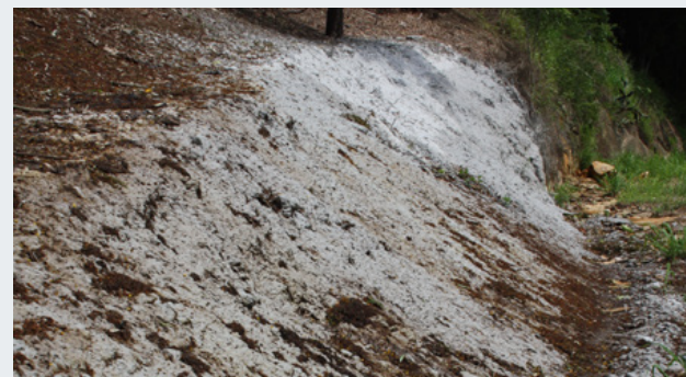
Post-Cyclone Oswald: January 2013
